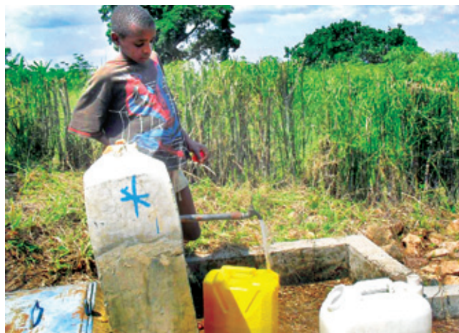
Gravity water now comes to the land and to the health centre
